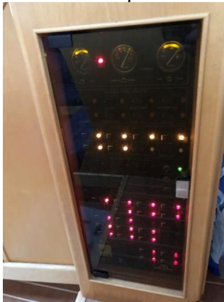
Electrical switch panel
